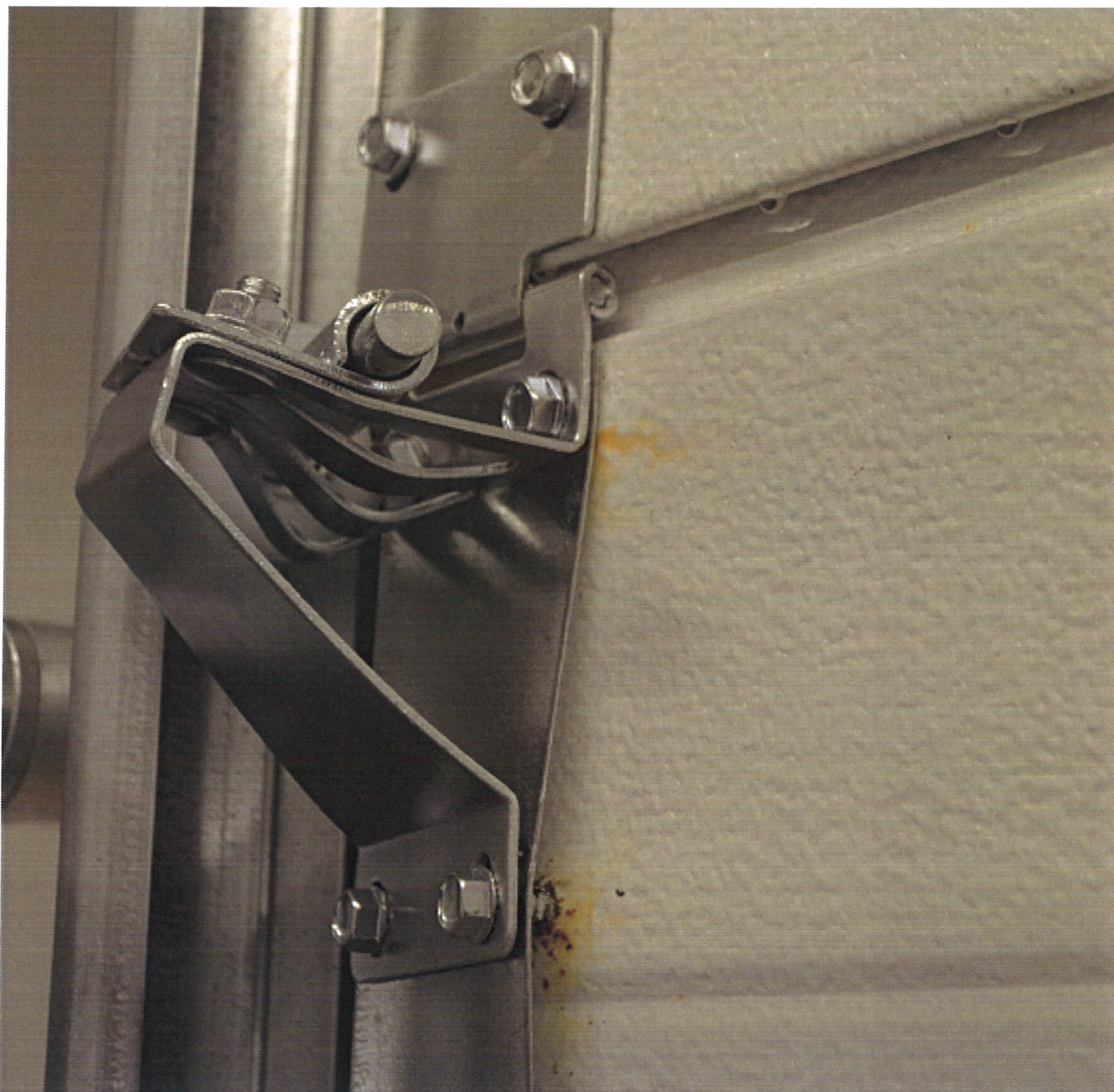
Figure 6. Deformation on the hinges after an inner pressure of about 900 Pa.
